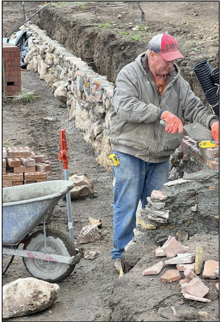
Ron Scherbarth working on the foundation of the greenhouse located on the Table south of Chadron.
